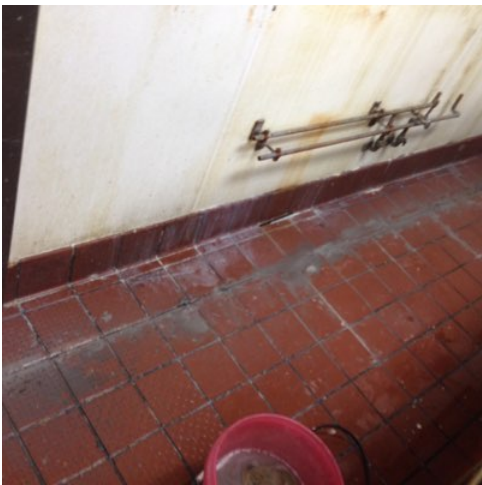
Photo 2 Pull dish machine and dirty dish table to access area.
