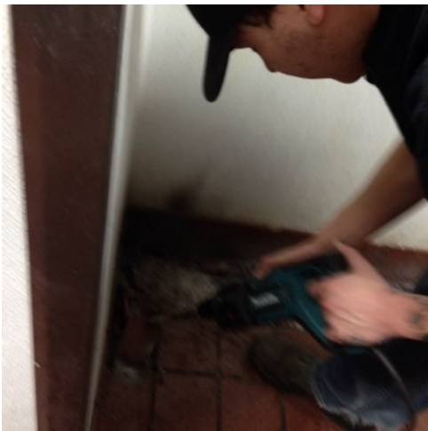
Photo 3 Using a hammer chisel, remove a roll of tile and base tile along wall.
